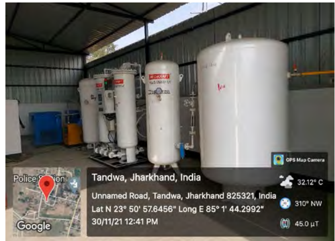
Oxygen Plant Chatra
